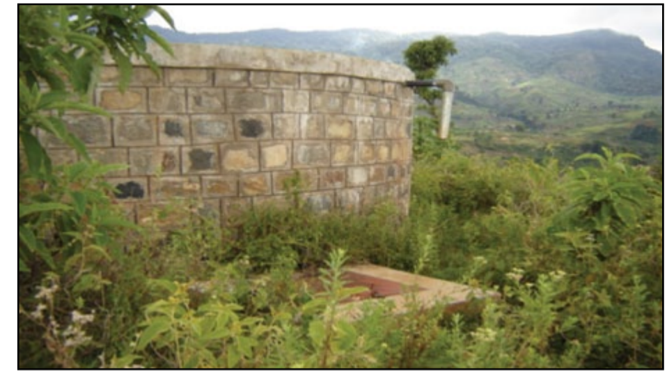
Water harvesting tank and reservoir
