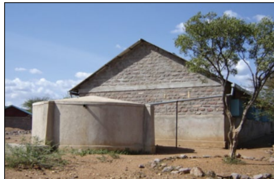
Rooftop rain water harvesting. In this case, rain water falls naturally down the slanted roof top to the gutters (the conveyance instrument) at the base of the roof. These gutters transport the water from the rooftop to the tank which is the collection devise. In the tank which is well constructed from cement, wire mesh and stones the water is safely stored here until it is used.
