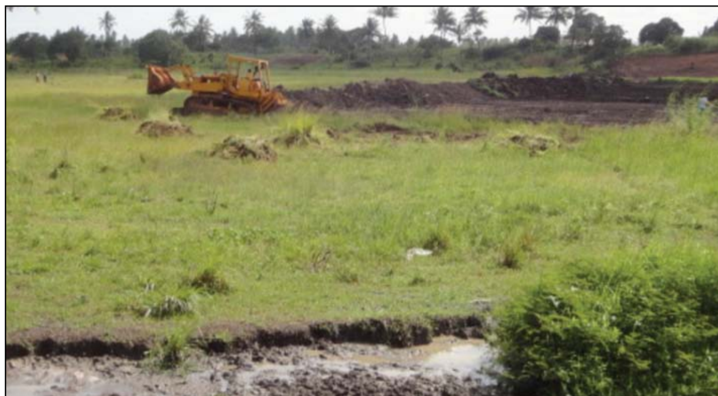
A KISCO bulldozer drilling a dam at Vidzyani on a section of the land in dispute between the company and the local community
