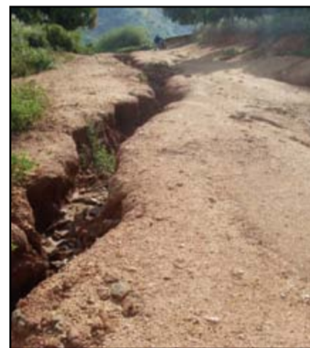
A section of a damaged road in the Kerio Valley region
