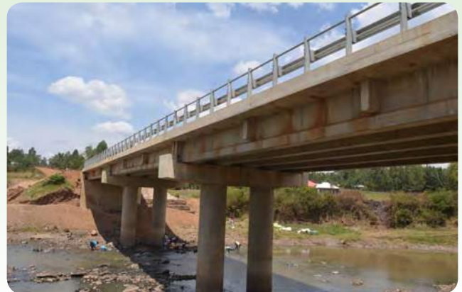
Kiringi Bridge that crosses River Migori in Migori town. The bridge was built by the County Government to decongest Migori town and also to ease trade and movements within the town
