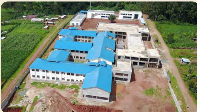
The modern Trans-Nzoia County Teaching and Referral Hospital under construction in Kitale town.
