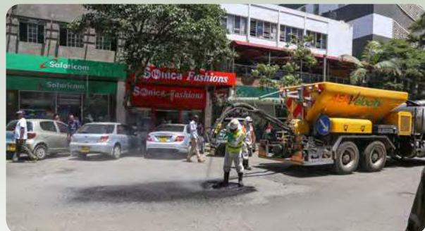
County staffs apply AEA-Patching technology to fill potholes along Kimathi Street. The technology is able to fill a typical pothole in between 3-5minutes.
