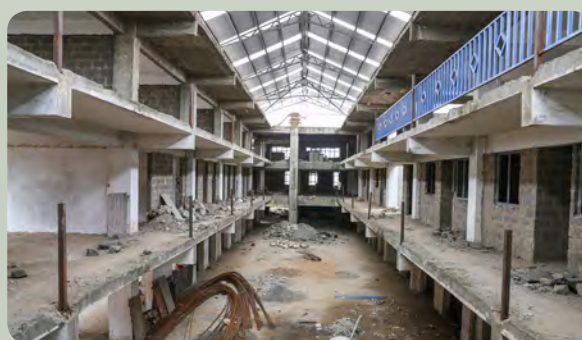
Ongoing construction of a three storey market in Westlands. The market will accommodate 384 small scale traders
