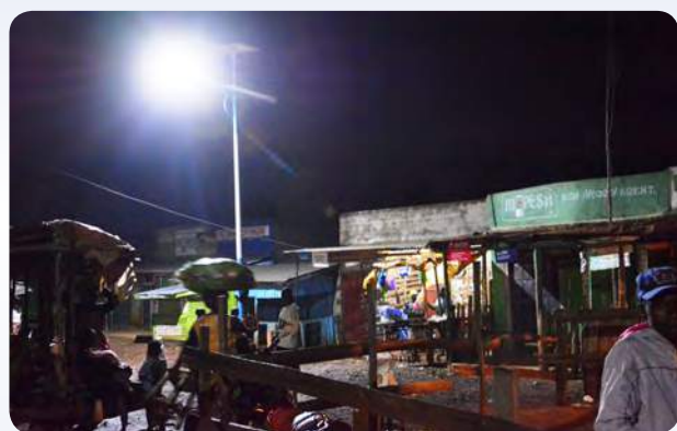
Traders sell their wares under solar street lights installed at Magena market, Bomachoge Borabu sub-county
