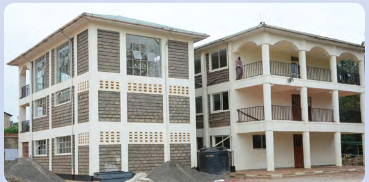
A section of the 250 bed capacity ward at Kisii Teaching and Referral Hospital. Upon completion, the bed capacity at the premier hospital will rise to 700 thus easing congestion.
