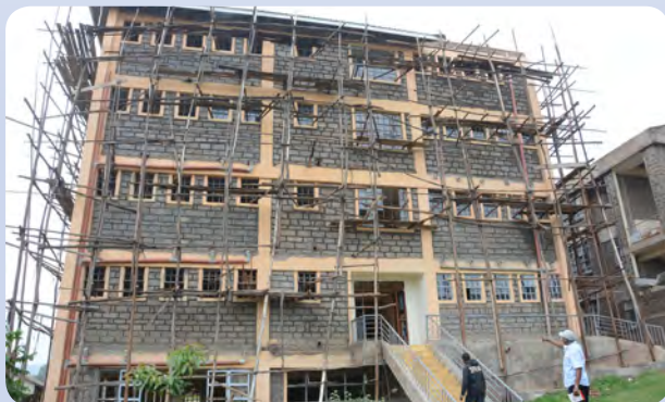
A section of the new 200 bed ward built by the County at the Kisii Teaching and Referral Hospital (KTRH). Once complete, it will increase bed capacity at the hospital to 700.
